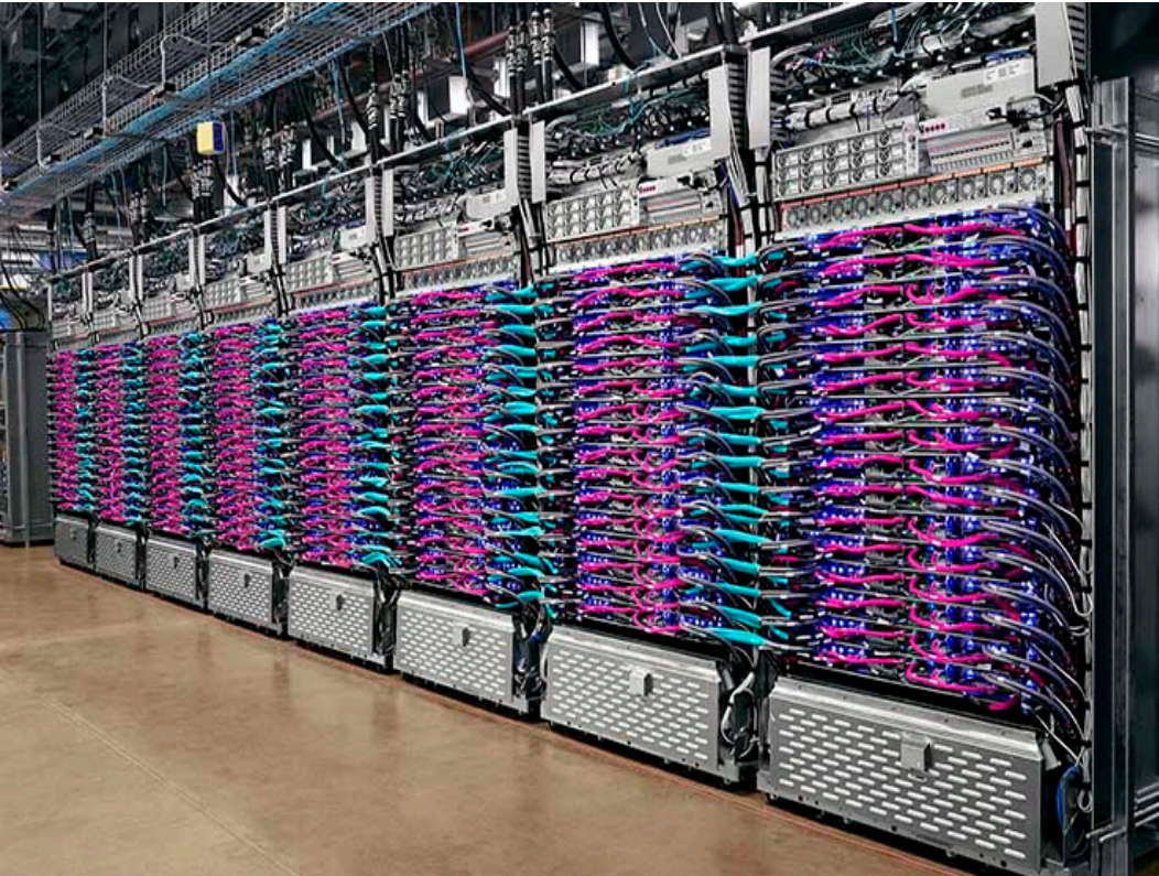
An eight-rack pod of Google's liquid-cooled TPU version 3 servers for artificial intelligence workloads
